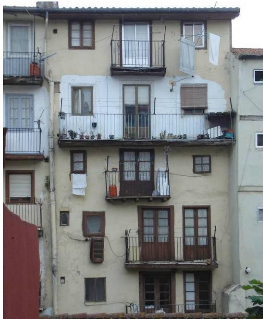
Fachada a consolidar
